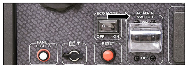
Figure 10 AC Main Switch
