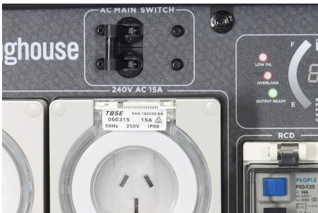
Figure 15 AC Main Switch in the ON Position
