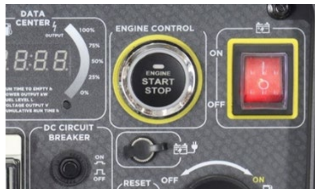
Figure 14 Battery switch in the ON Position
