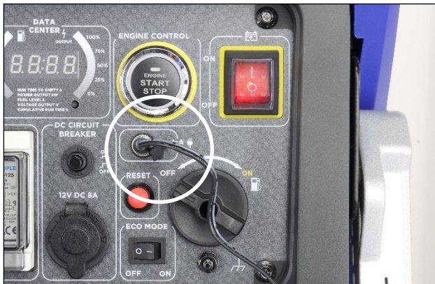
Figure 34 Connecting the Battery Charger to the Generator
