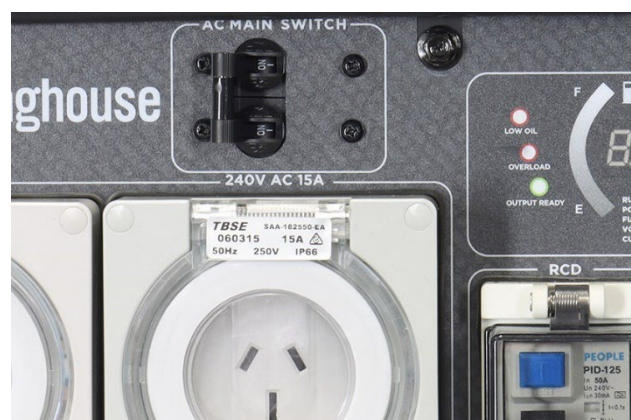
Figure 15 AC Main Switch in the ON Position
