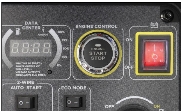
Figure 14 Battery Switch in the ON Position
