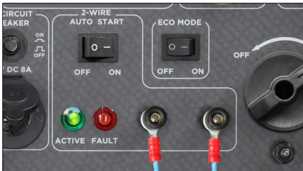
Figure 19 2-Wire Auto Start Panel
