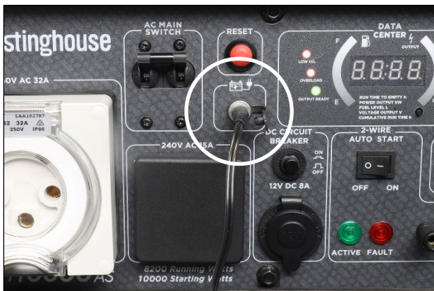
Figure 34 Connecting the Battery Charger to the Generator
